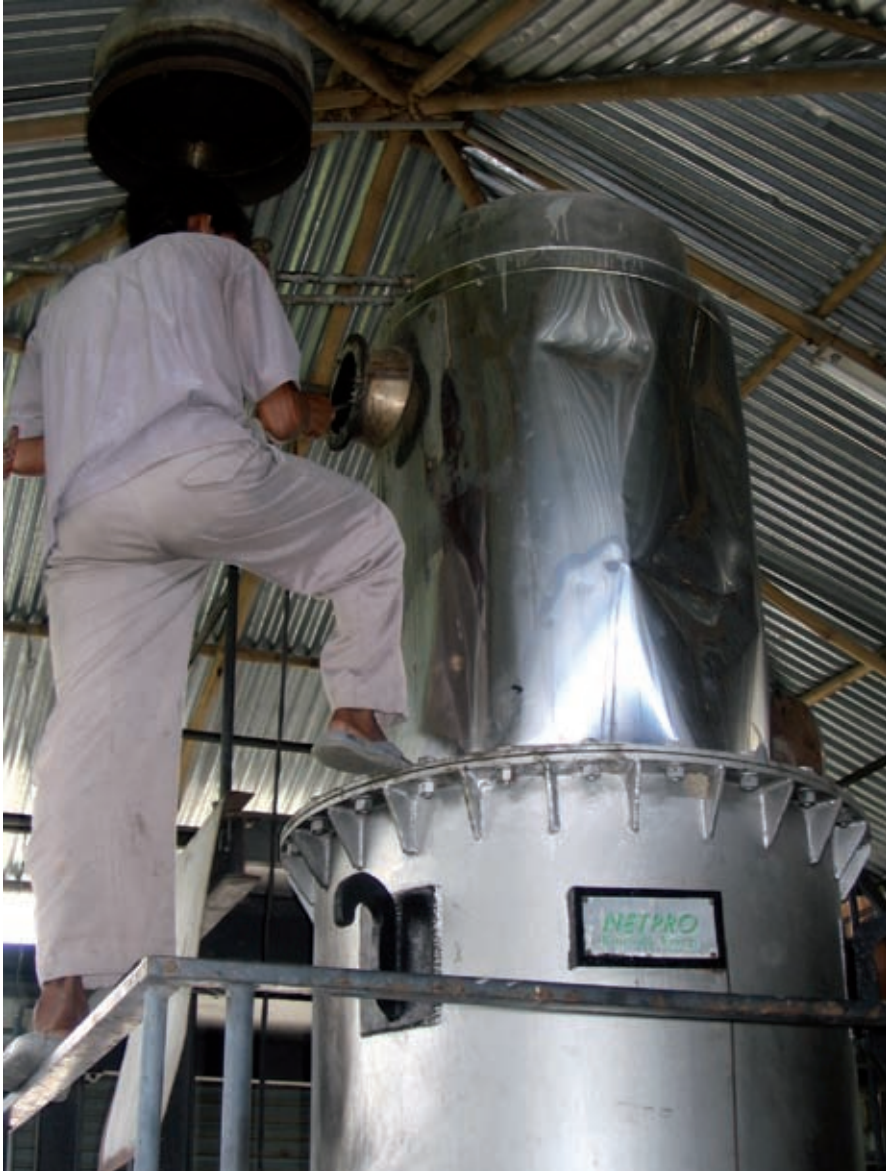
Maintenance in the biomass gasifier in Baharbari, India (2006)
