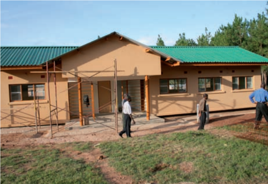
Construction of new classrooms, St. Johns upper basic school, Mungwi, Northern Province.
